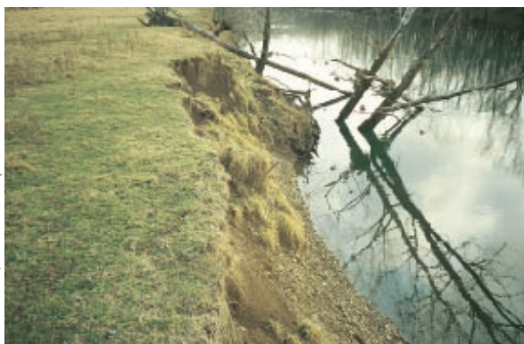
Figure 2. Bank sloughing is a dangerous form of instability that requires attention to the base or toe of the slope. Planting trees at the top of the bank would only worsen the condition.
