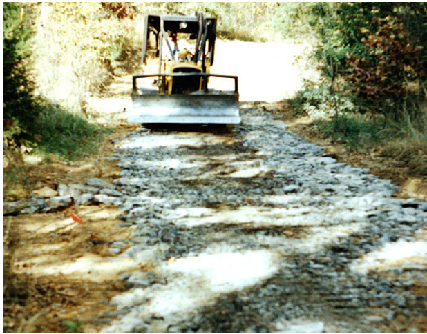
Figure 7b. Dozer leveling rock fill. Lower end wall and apron have been completed.
