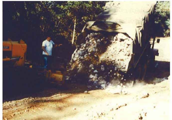
Figure 4d. Additional fill in channel
