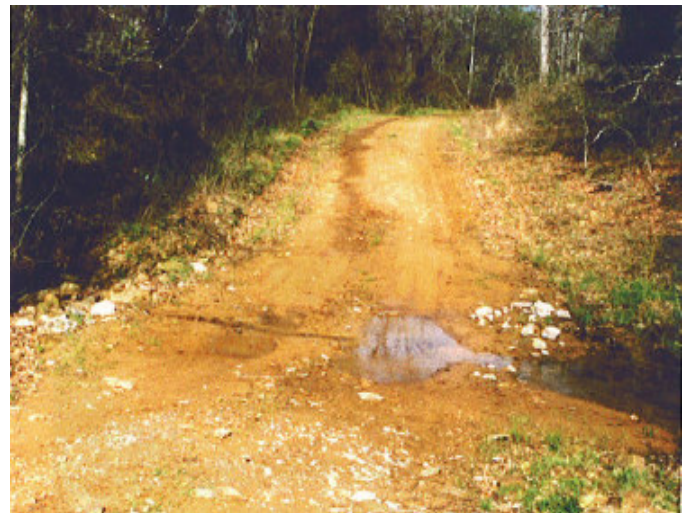
Figure 4f. The ford two years following completion and with heavy log truck use
