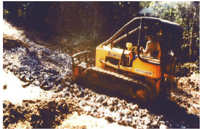
Figure 4e. A dozer leveled and shaped the rock fill to form the roadway surface
