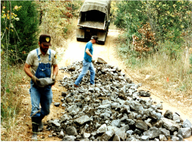
Figure 7a. Rock fill on a wide, flat crossing on an old road. The end wall is being placed by hand.
