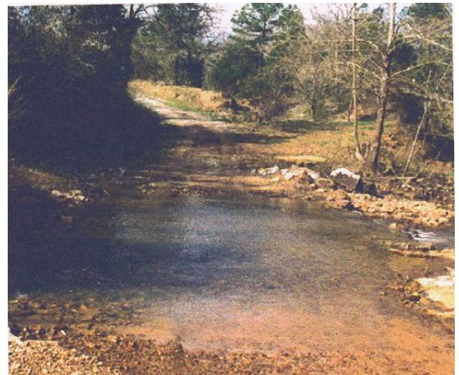
Figure 12. Completed Clear Creek ford with upper and lower end walls (looking toward the south approach)
