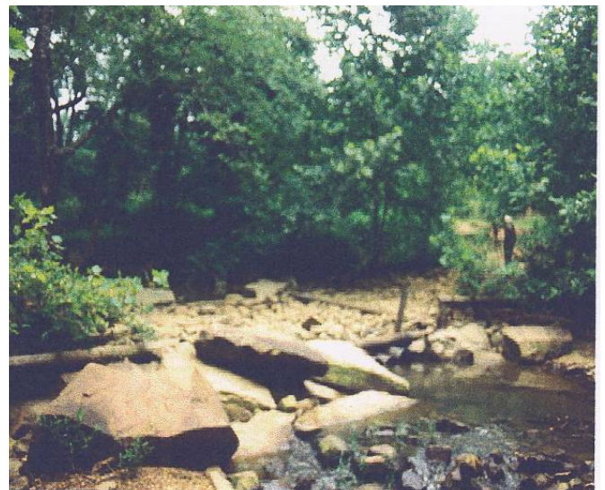
Figure 4a. Washed-out part of previous rocked ford on Caney Creek (note the pole cribbing)
