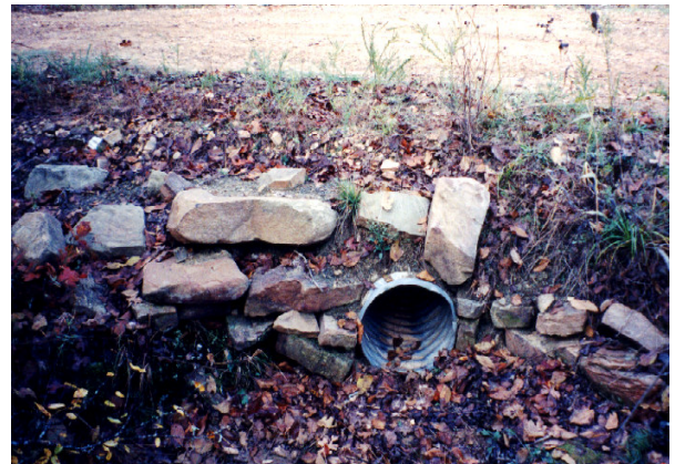
Figure 7. Where fast runoff water is expected, protect the inlet with larger rock.
