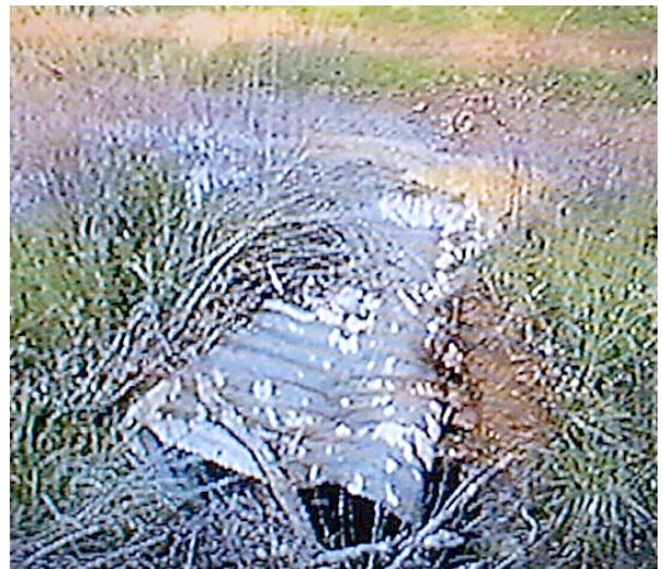
Figure 3. Insufficient fill leads to a flattened culvert.
