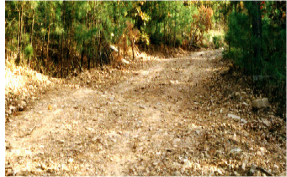
Figure 3. Where dip height is too low, high water may flow over the berm and cause erosion
