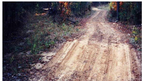
Figure 5. The trough of the dip is filling in because of too little slope (less than 3% average)
