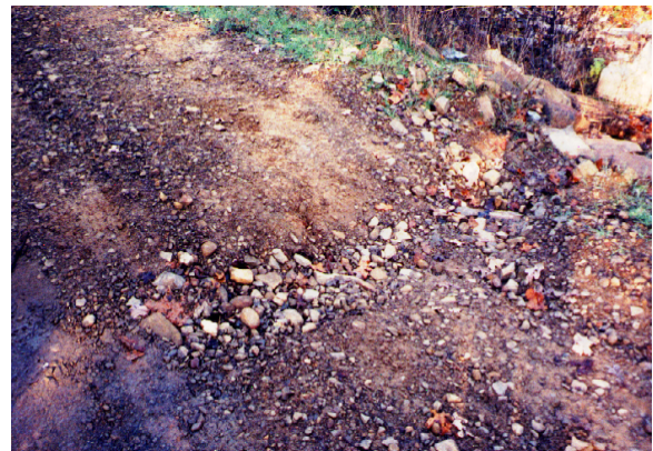
Figure 4. The trough of the dip is eroding because the slope is too steep (over 3% average)
